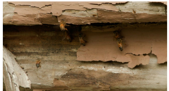
Once a bee swarm has established itself inside a wall or structure, it can be difficult to remove.
