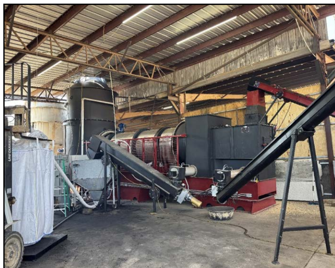
Figure 3. Small-sized Biochar production facility located in Arkansas. Photo by Sagar Chhetri.
