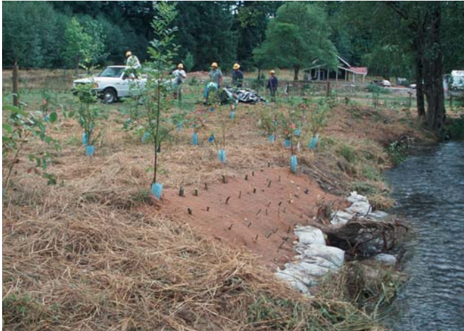
FIGURE 4. A streambank stabilization project at various stages of plant growth with cost-share funding through the Wildlife Habitat Incentives Program (WHIP).
