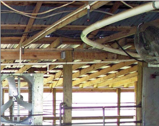
Figure 4. When hanging sprinklers, consider electrical wiring, rafters and other items affected by the sprinklers. Sprinklers that face up will not drain water when they are not under pressure from the pump unless the slope is great enough to allow the end sprinklers to be lower than the initial sprinklers.
