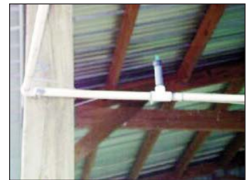
Figure 9. Sprinklers that point up maintain pressure and fill more quickly than sprinklers pointed down.
