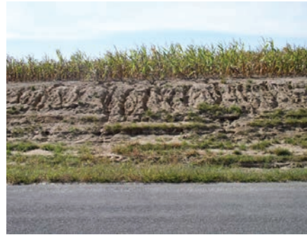
Figure 2. Soil erosion along a ditchbank lacking grass groundcover. (Photo from www.in.gov )
