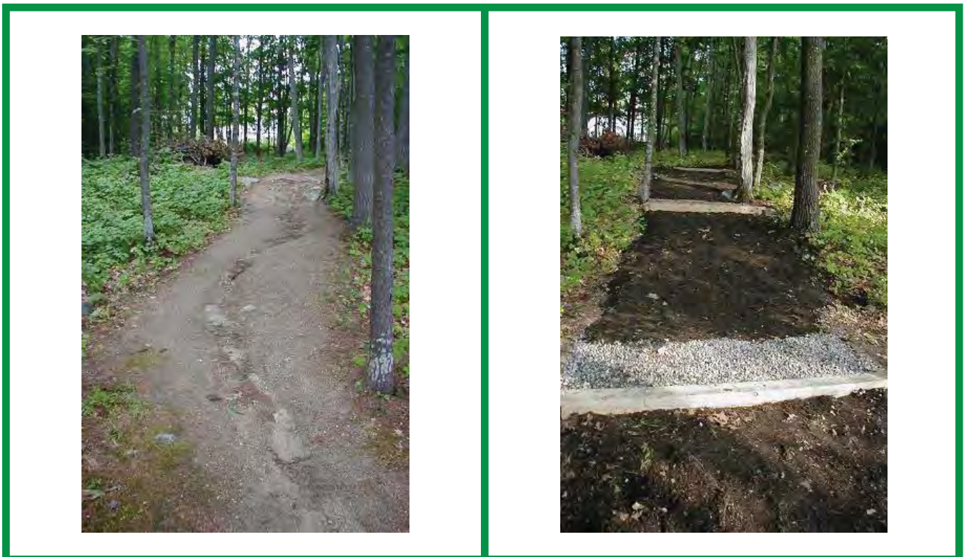
FIGURE 17. Trail before and after waterbars were installed to divert water off the tread. Waterbars should be installed only as a last resort. Photo courtesy of Maine Department of Environmental Protection, Bureau of Land and Water Quality.
