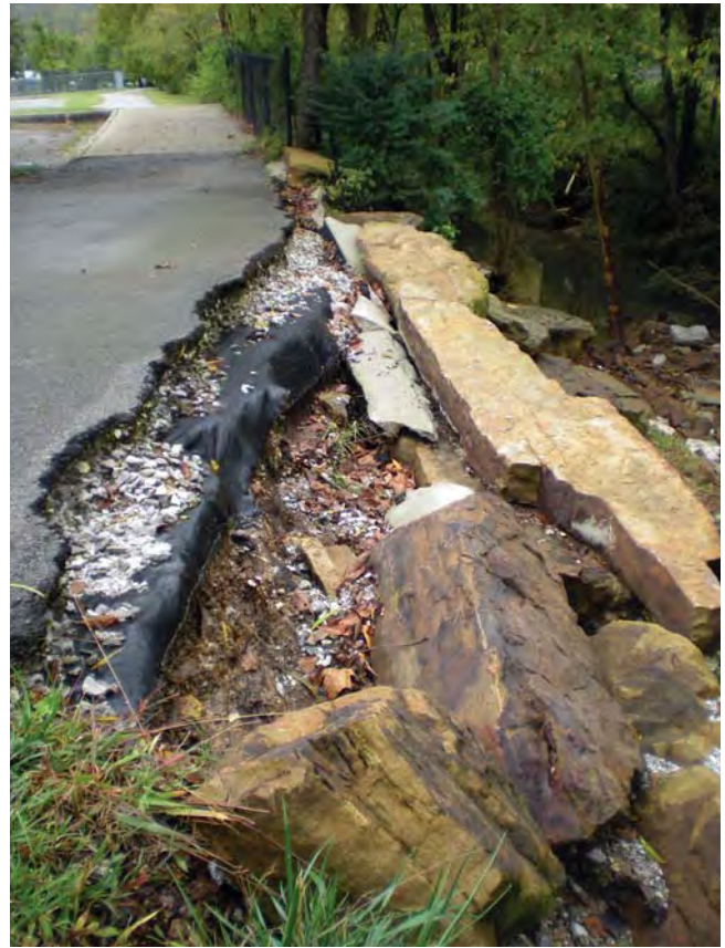
FIGURE 6. This trail was built too close to the stream. Buffers reduce soil erosion, improve water quality and provide habitat for wildlife. Photo by John Pennington, UA Division of Agriculture, Cooperative Extension Service.
