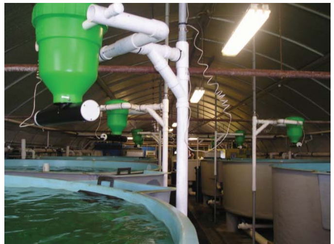
FIGURE 9. Recirculating systems require careful attention. (Photo by Paul Willis)
