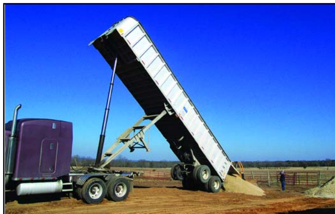
Blend of bottom ash and fly ash being delivered to the heavy use area. The existing top layer of manure and mud has already been removed and land applied.
