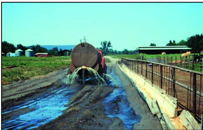
Watering of mixture of fly ash and soil during placement and compaction.
