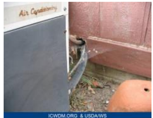
A gap around the central air pipe allowed rodents to enter this home. Photo by Stephen Vantassel, www.icwdm.org .
