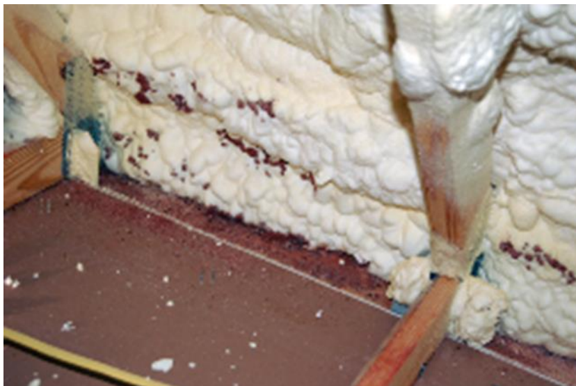
Spray foam insulation can hide termite activity. Termites can build mud shelter tubes near, on and through spray polyurethane foam insulation. Photo courtesy of Jim Fredericks, National Pest Management Association.
