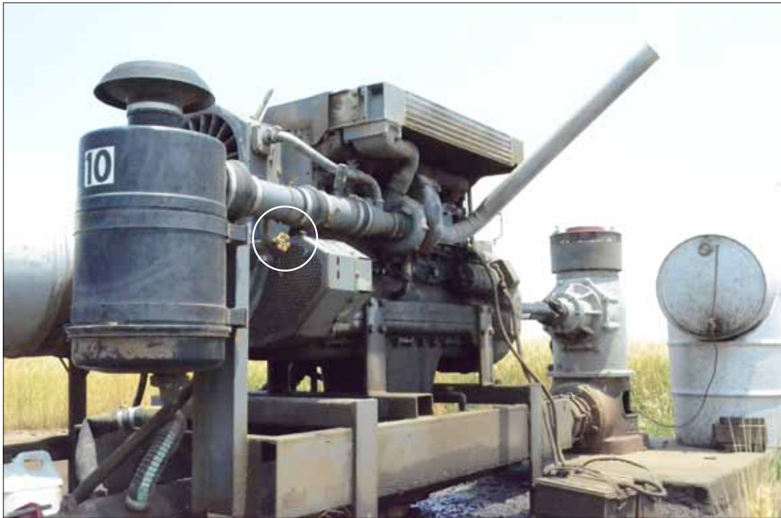
At this dual fuel pumping plant, natural gas is injected along the intake line just prior to the turbocharger and regulated by a gate valve. (Notice the yellow valve handle in the middle of the photo marked with a white circle.)
