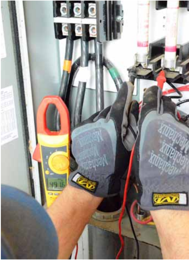
Testing voltage with Fluke 336 True-RMS clamp meter.
