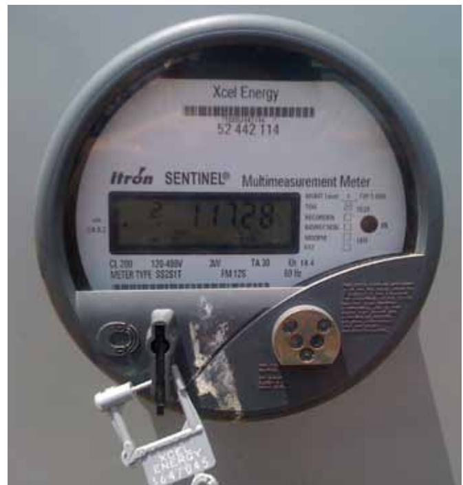
Typical digital electrical meter.
