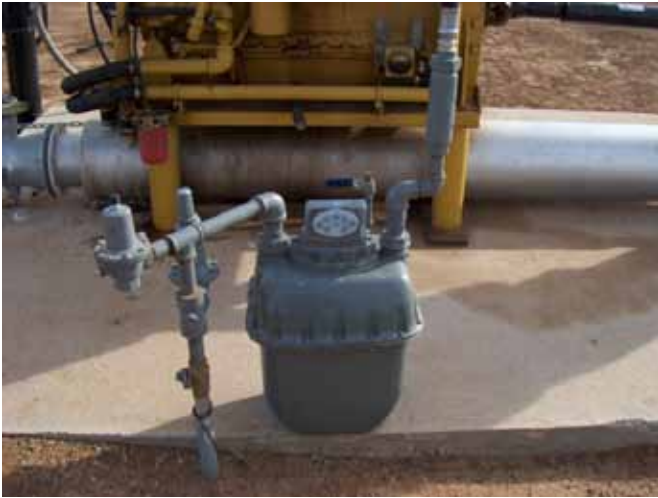
Rockwell No. 750 diaphragm gas meter. From left to right, notice the isolation valve, regulators, meter, 1/4 inch port with ball valve and inline gas filter.
