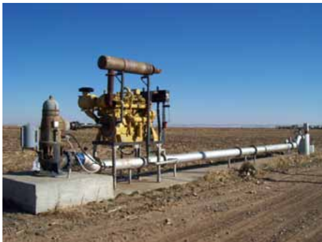
Caterpillar 3406 - TA natural gas pumping plant.
