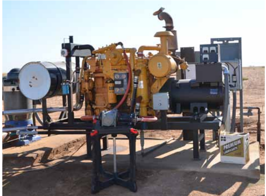
Natural gas Caterpillar 3306TA driving a Marelli three-phase generator, providing power to three irrigation wells.
