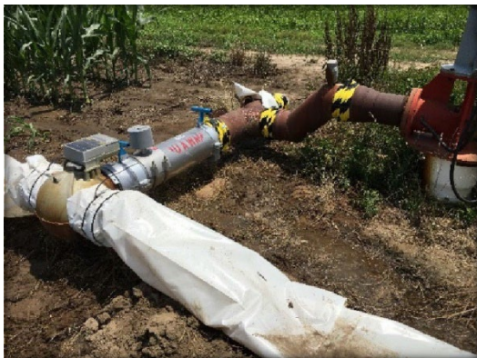
Figure 1. Example of Universal Hydrant Sealing
