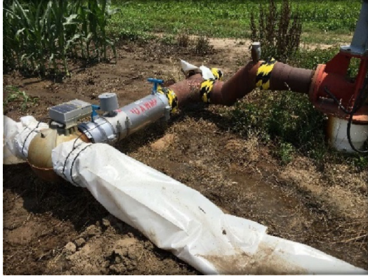
Figure 1. Example of Universal Hydrant Sealing
