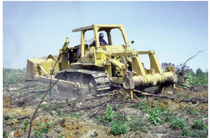
Figure 3. Ripping contracts must be carefully written to minimize the risk of site damage.
