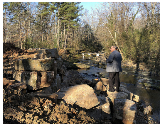
NEARLY COMPLETE Dr. Rick Cartwright surveys the bank stabilization project at the Little Rock State Extension Office on Dec. 21, 2018. The project is nearing completion.
